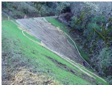
Slide Repair on Chamise Road
