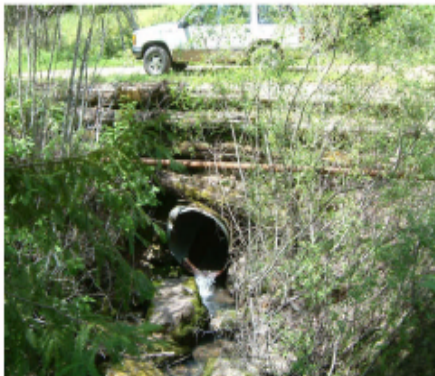
DOWNSTREAM SIDE OF THE CURRENT STREAM CROSSING SHOWS A CONFINED CHANNEL AND A CULVERT THAT IS NOT ALIGNED WITH THE ROAD.
